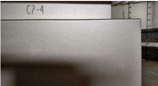
Figure 7: Each panel or assembly is identified with a permanent ID number which corresponds to its location on the building and is coordinated in the shop drawings.
